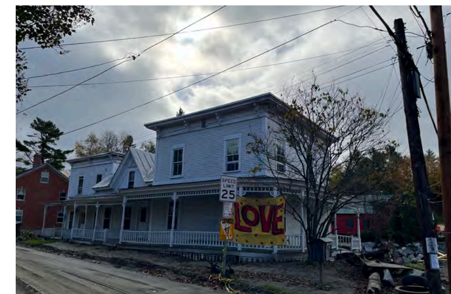
A property rendered uninhabitable by the flooding Image Source: Planning Team
